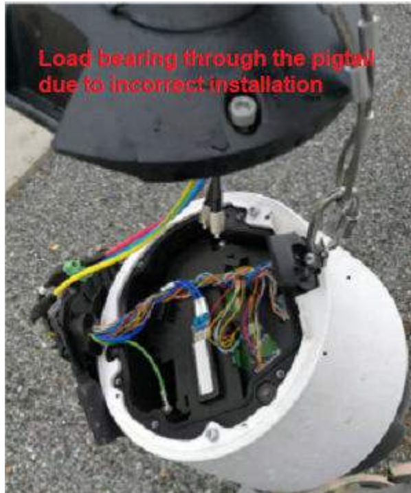
Figure 3-24 Load bearing through the pigtail due to incorrect installation
