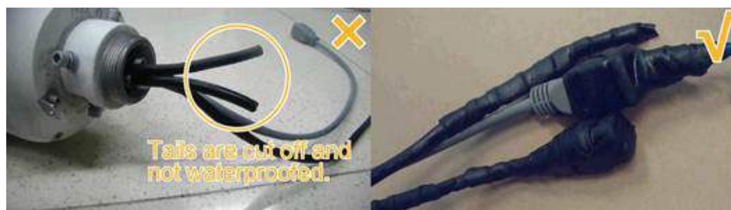
Figure 3-1 The pigtail is cut off and is not waterproofed.
