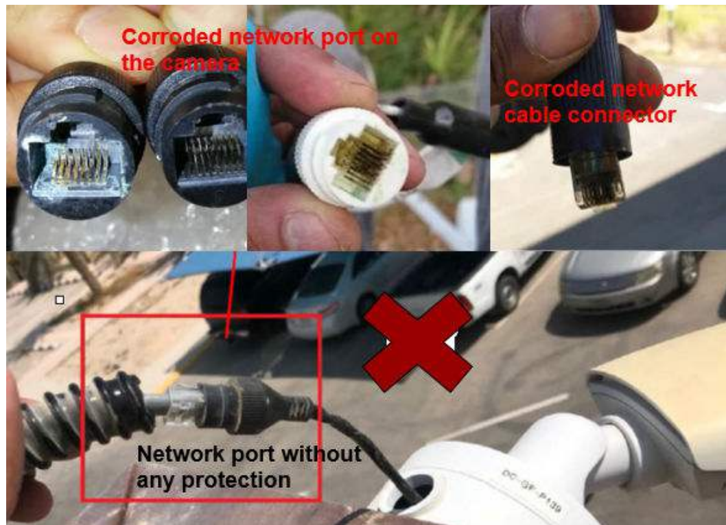
Figure 3-20 Corroded network ports and connectors
