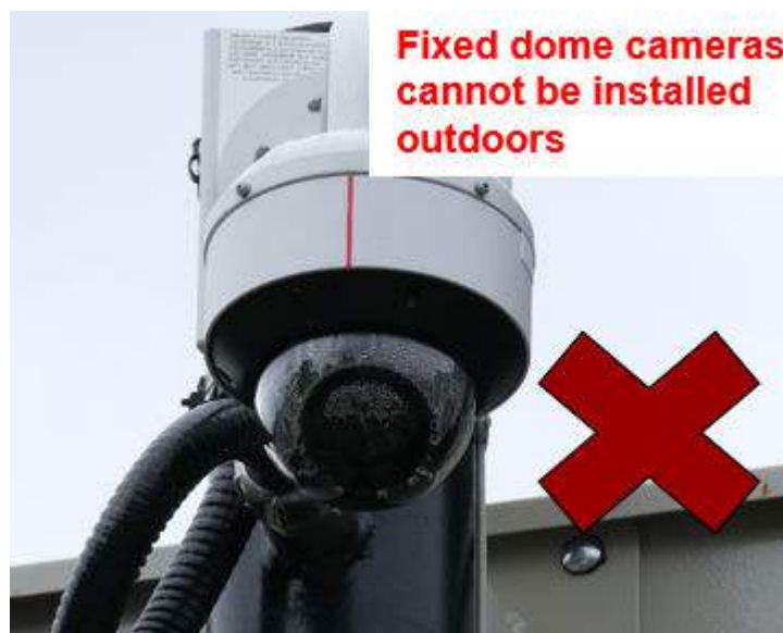
Figure 3-31 Outdoor installation of the fixed dome camera
