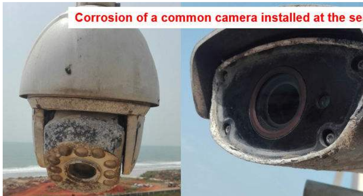
Figure 3-38 Corrosion of a common camera installed at the seaside
